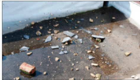
Fredericksburg No. 4 roof damage
